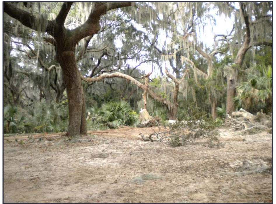
Former Cattle Dip Vat, St. Simon's Island November 2014 Used local soil to backfill excavation
